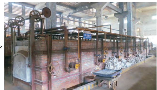
焙烧炉 Roasting Furnace
