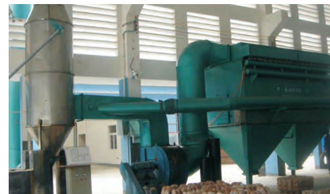
焙烧炉 Roasting Furnace
